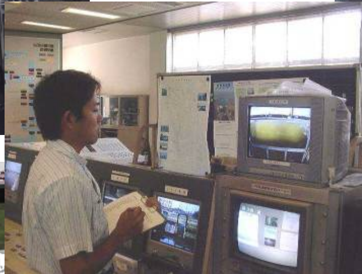
Operation-room (Monitor & Operation)
