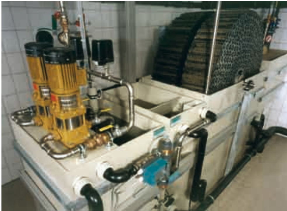
Figure 4: Rotating biological contactor (RBC) for greywater treatment in Hannover, Hågewiesen (Photo: B. Ebeling)
