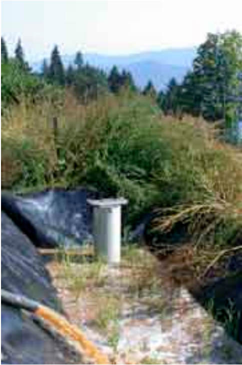
Figure 3: An STRB for primary sludge from a 3-chamber septic tank of a 32 pe RBTS ("Weissmann" demonstration site)
