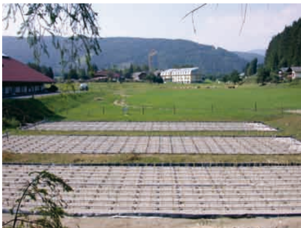
Figure 1: Fischerhof constructed wetland for 160 pe, Sirnitz/Austria
