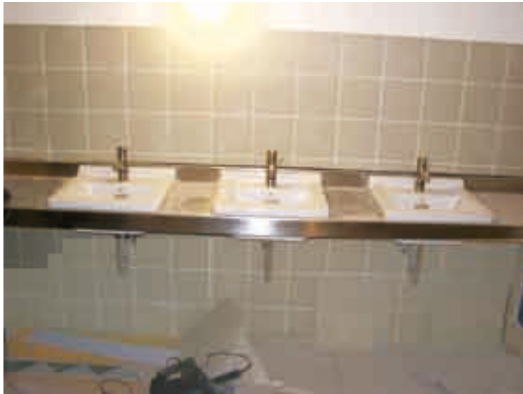
Figure 4: Ceramic sinks in a stainless steel washstand with vacuum connection at Burg Lenzen
