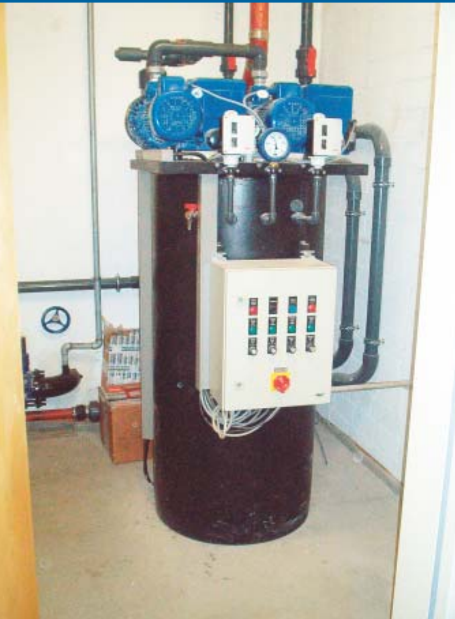
◀ Fig. 1: COMPACT VACUUM STATION WITH TANK, VACUUM PUMPS, DISCHARGE PUMPS AND CONTROL PANEL AT A SOLAR PANEL FACTORY AT BRAUNSCHWEIG, GERMANY.
