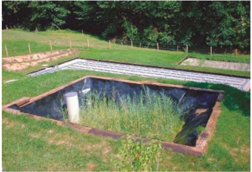
Fig. 3: SLUDGE TREATMENT REED BEDS (STRB) FOR PRIMARY SLUDGE FROM A 3-CHAMBER SEPTIC TANK OF A 50 PE CONSTRUCTED WETLAND PLANT
