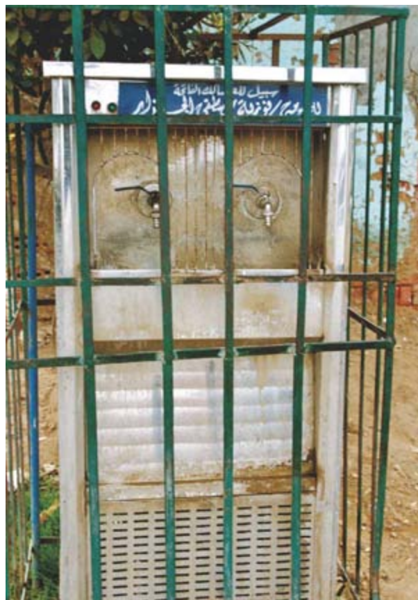
Fig. 2: A NEWLY INTRODUCED ELECTRIC WATER COOLER OUT OF OPERATION (NILE DELTA)
