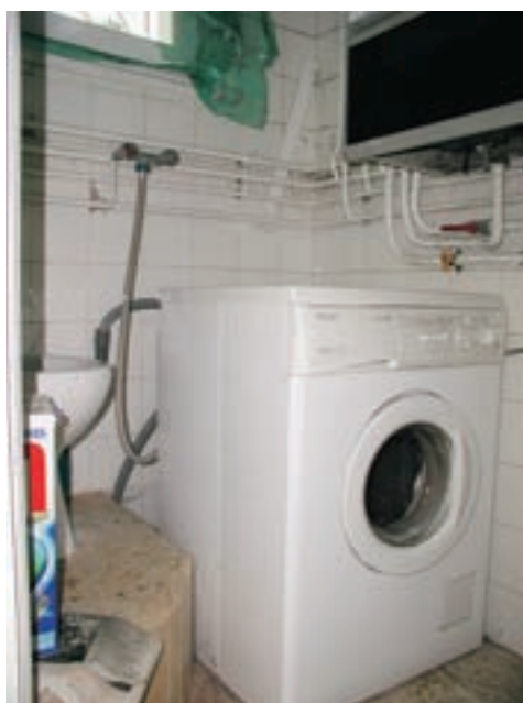
Fig. 11 WASHING MACHINE CONNECTED TO A RAINWATER CISTERN IN A PRIVATE HOUSE
