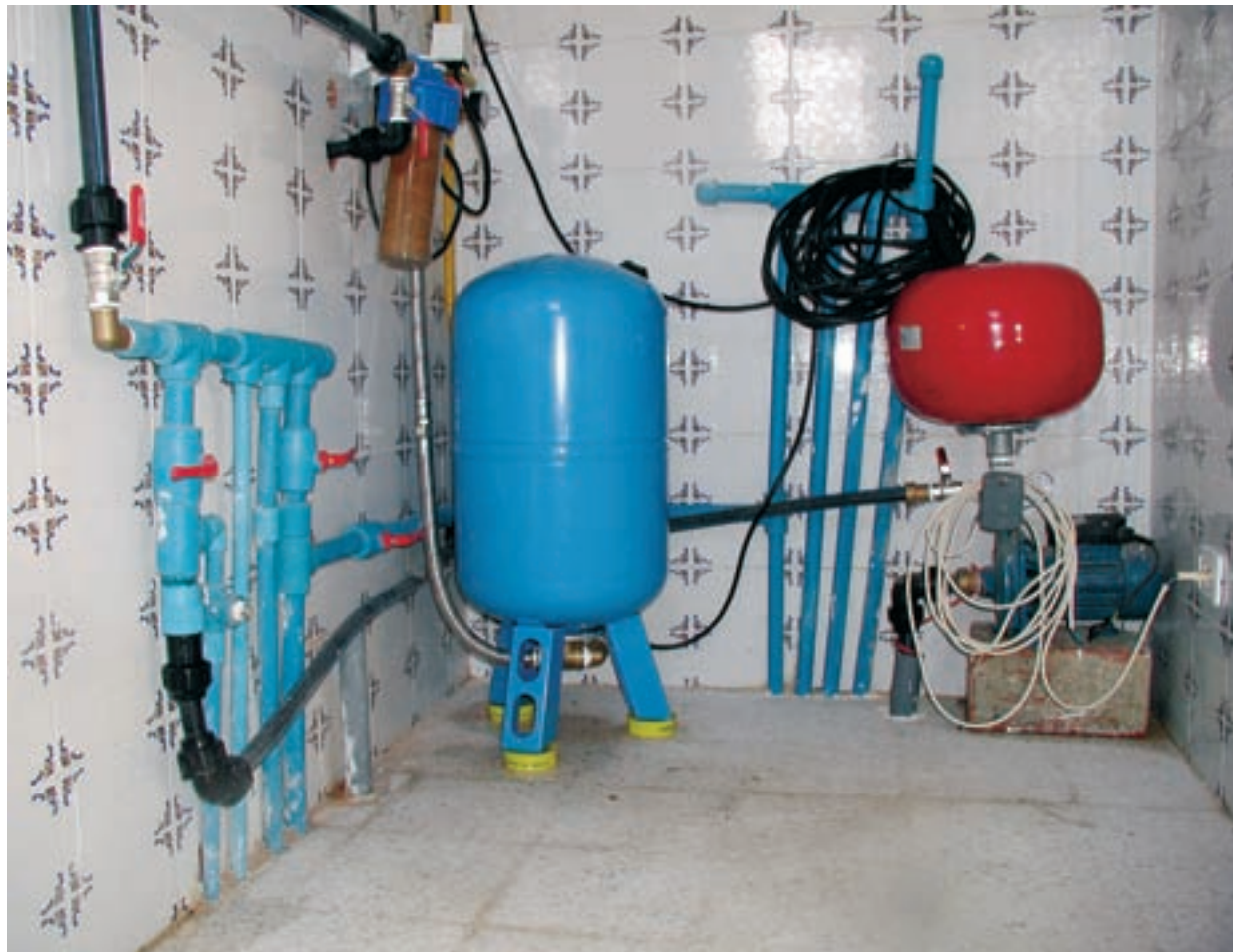
Fig. 5 COMBI SYSTEM FOR RAIN WATER AND WELL WATER USE IN A RESIDENTIAL BUILDING IN TUNIS, TUNISIA
