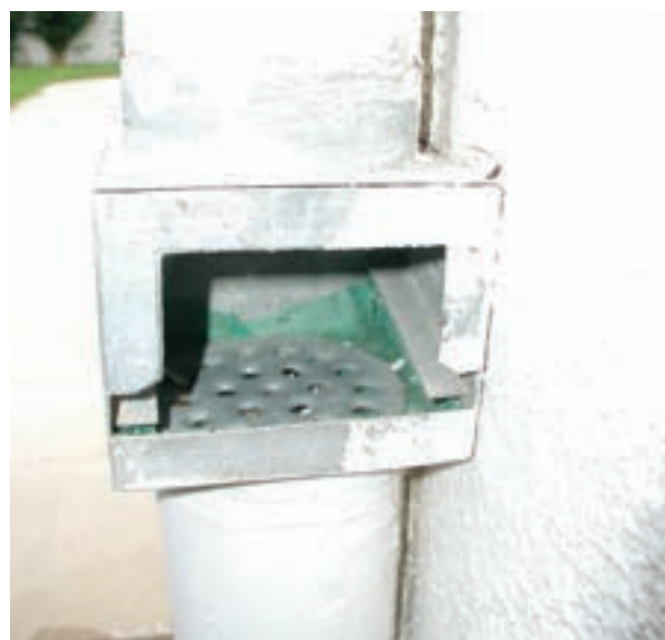
Fig. 5: TRADITIONAL FILTER FOR HARVESTING RAINWATER INSERTED IN THE PIPE
