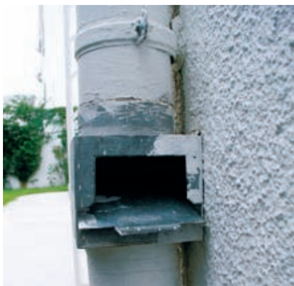
Fig. 9: TRADITIONAL FILTER FOR HARVESTING RAINWATER, POSITION FOR ELIMINATION OF THE FIRST FLOW
