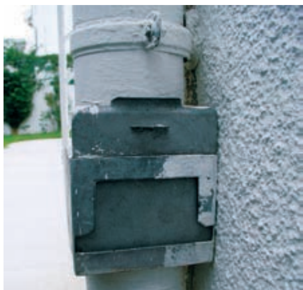
Fig. 8: TRADITIONAL FILTER FOR HARVESTING RAINWATER, POSITION FOR FEEDING THE CISTERN
