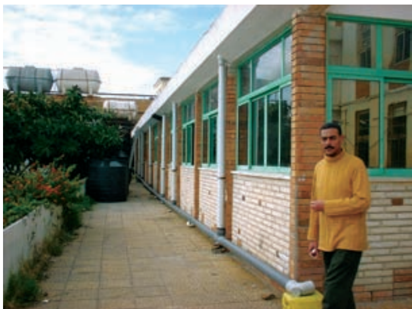
Fig. 3: CONSTRUCTION OF A RAINWATER HARVESTING SYSTEM AT THE OCEANOGRAPHIC INSTITUTE IN ALEXANDRIA, EGYPT
