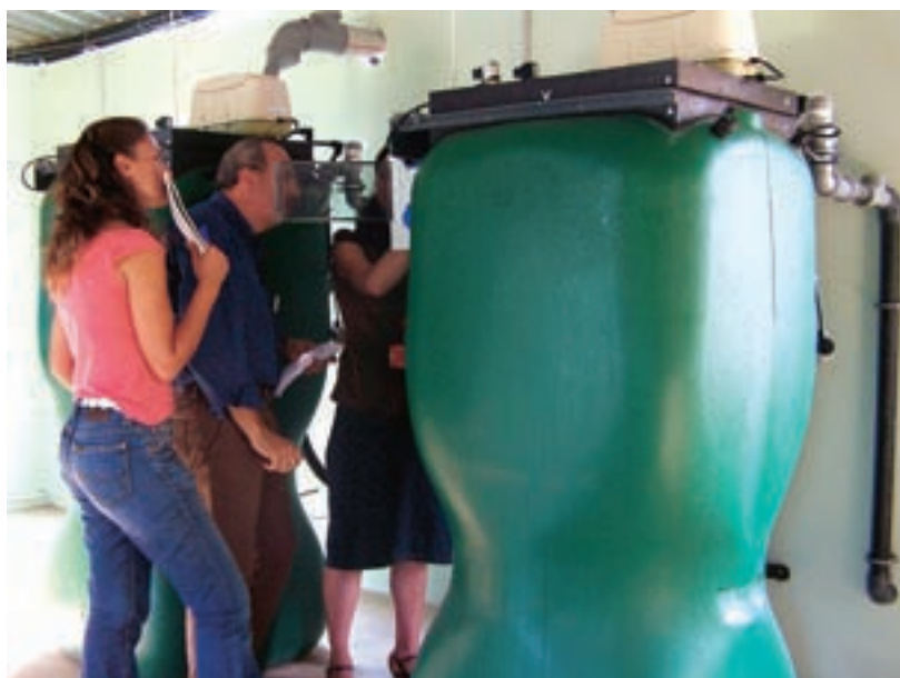
Fig. 1: COMMISSIONING OF MEMBRANE BIO-REACTORS AT THE TURKISH TDC, MARMARA RESEARCH INSTITUTE IN GEBBZE
