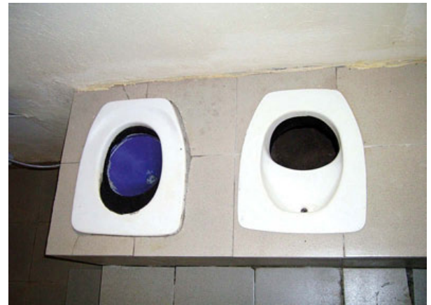
Fig. 5: DESIGN FOR A SEATER URINE DIVERTING DRY VAULT TOILET. ONE SEAT FOR URINE AND FAECES (RIGHT SIDE) AND ONE FOR ANAL WASHING (BURKINA FASO)
