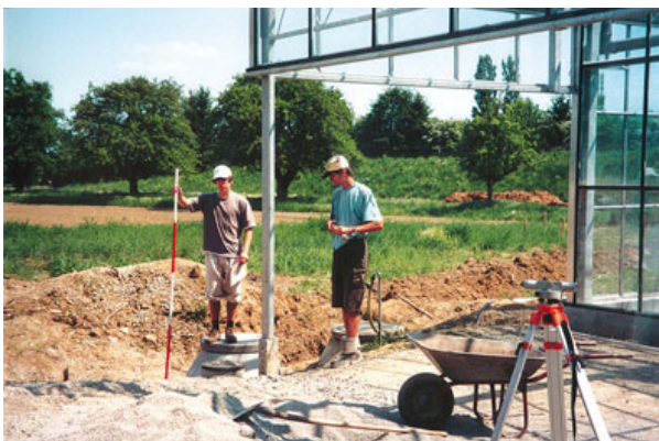
Fig. 5: STUDENT BUILDING IRRIGATION SYSTEM WITH RAINWATER AT STEINER SCHOOL
