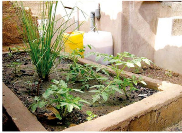
Fig. 6 + Fig. 7: ANAL WASHWATER DRAINED TO A SOAKAWAY (LEFT) AND EVAPO- TRANSPIRATION BED (RIGHT) IN MALI
