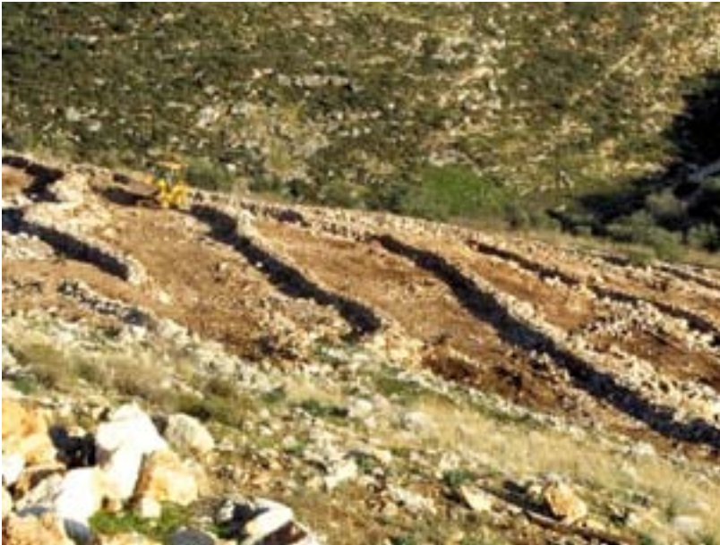
▲ Fig. 2: TERRACING MODE FOR RAINWATER HARVESTING
