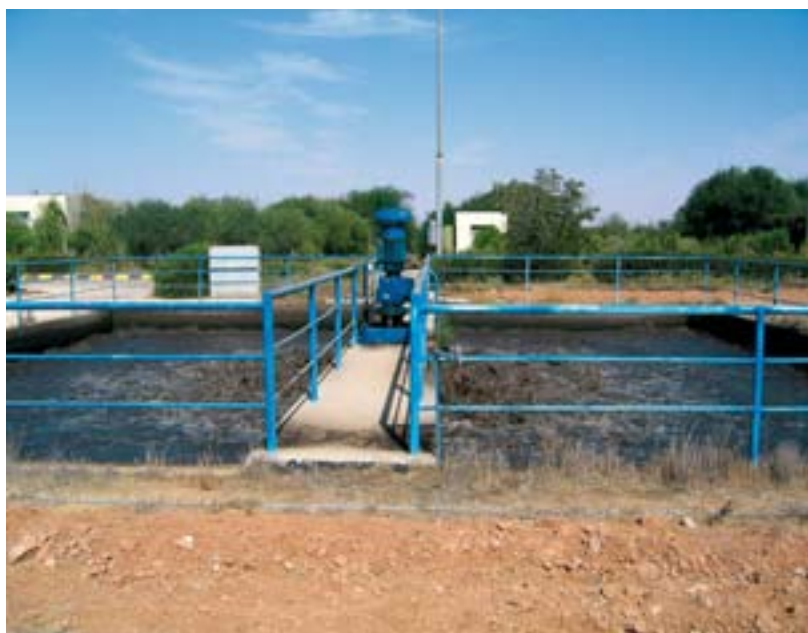
▼ Fig. 4: SMALL WWTP AT THE AL AL-BAYT UNIVERSITY CAMPUS, AL MAFRAQ, JORDAN
