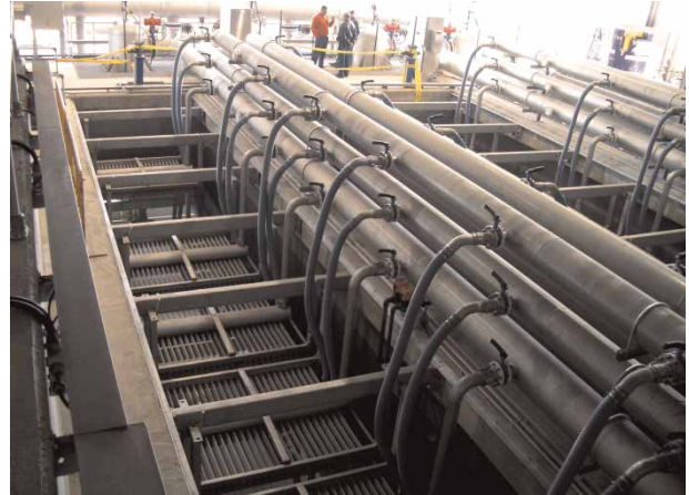
Figure 3 | Detail of San Pedro treatment plant.
