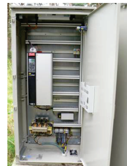
Figure 17: Pump with variable frequency drives at water collection well
