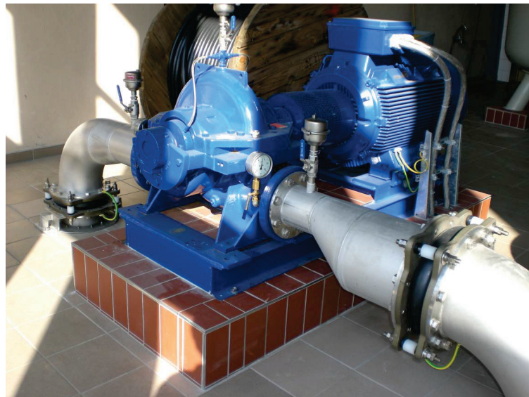
Figure 18: Frequency driven pump
