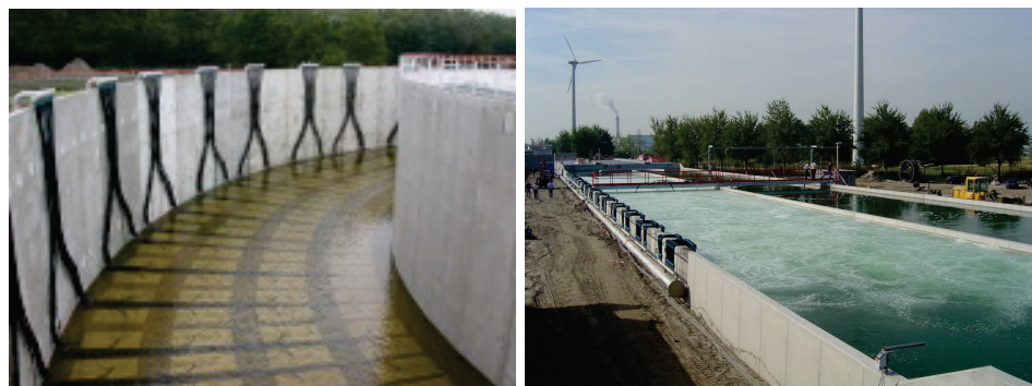
Figure 20: Plate aerators at bottom of wastewater treatment aeration tank
