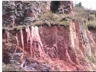
Sandstone to infiltration of water
