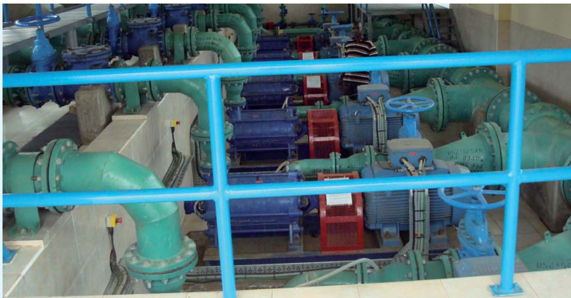
Water Pumping in Nakuru, Kenya
