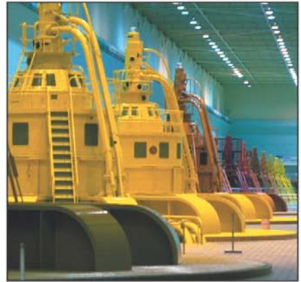
Generators at The Dalles Dam (OR)
